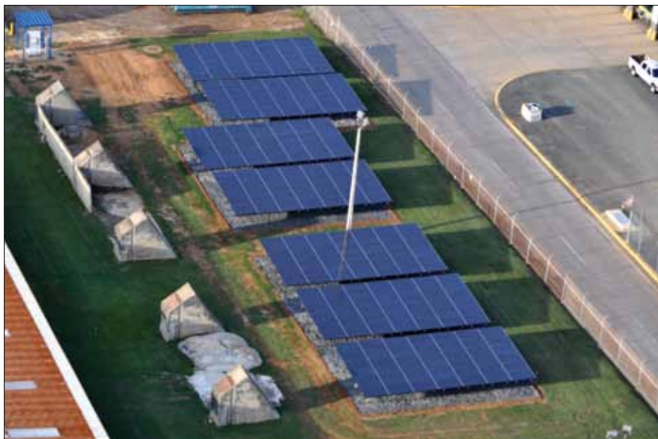
The service recently installed solar panels at Air Station Borinquen. [Photo courtesy of U.S. Coast Guard]
